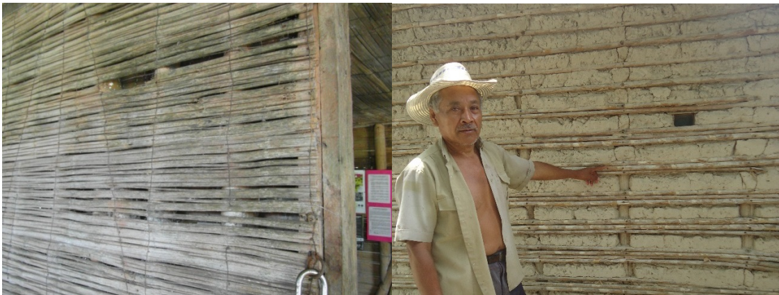
Figure 3. Typical wall matrices for traditional bahareque (Kaminski, 2016): (L) esterilla/caña picada (sheets of bamboo formed by splitting bamboo along its length and then unrolling it; (R) caña brava/vara de castilla (small diameter bamboo/cane).
